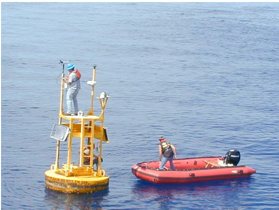
TABS 2.25. being repaired after a ship tied up to it breaking a solar panel and wind sensor
